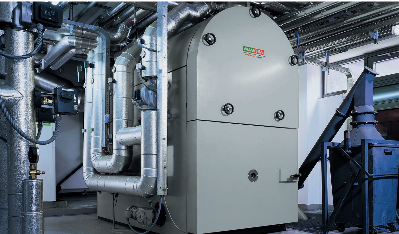
2 × palenisko podsuwowe FU 2500 RA, Mosser Leimholzbau, Randegg, AT
